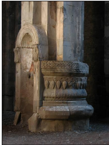
Fig. 2. Church of St John the Baptist in Oskhi. Interior. Niche in the south-west pier of the dome
