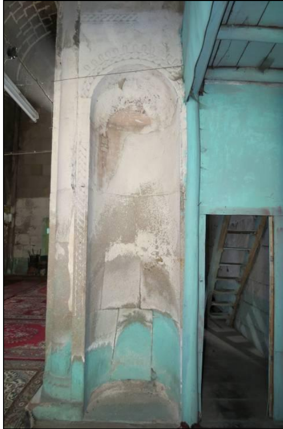
Fig. 5. Church of the Mother of God in Khakhuli. Interior. Niche in the north-west pier of the dome
