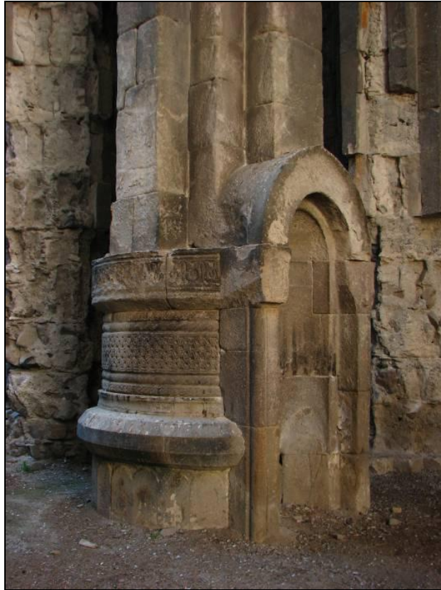
Fig. 4. Church of St John the Baptist in Oskhi. Interior. Niche in the north-west pier of the dome
